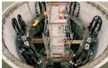
6 th Bridge of Rouen, France Lowering by about 15m of four 3,000t concrete caissons and two 2,400t foundations into the River Seine for the 175m-high bridge pylons.
