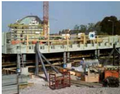
Bridge over Werkkanal, Bürglen, Switzerland Lifting and lowering of a 500t bridge deck by means of jacks and packers.
