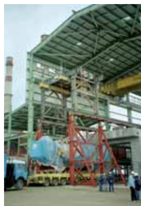
Severnaya 400 MW CCPP, Baku, Azerbaijan Positioning of a gas turbine and generator, each of 350t, required lifts of 15m and sliding by 60m. Twelve HRSG boiler modules of 1,700t total weight were also lifted.
