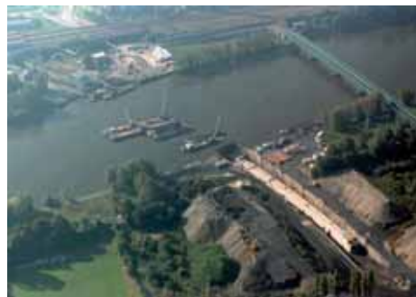
Tunnel under Vltava River, Prague Metro Line C, Czech Republic Underwater pulling of a 168m-long concrete tunnel in a pre-excavated trench. Tunnel weight: 6,700t
