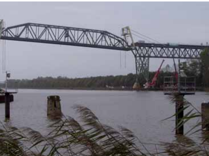
Railway Bridge Hochdonn, Germany Replacement of the centre span weighing 1,465t. Lowering/lifting 40m combined with tilting movements to preserve the original supports.
