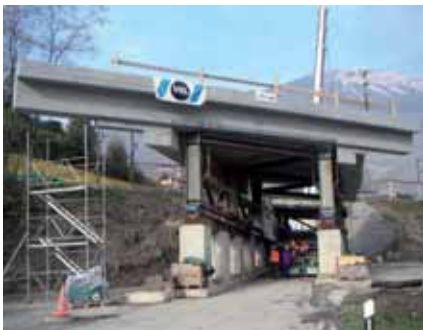
Salgesch Railway Bridge, Sion, Switzerland Lifting, sliding and lowering of the 400t superstructure onto its abutments
