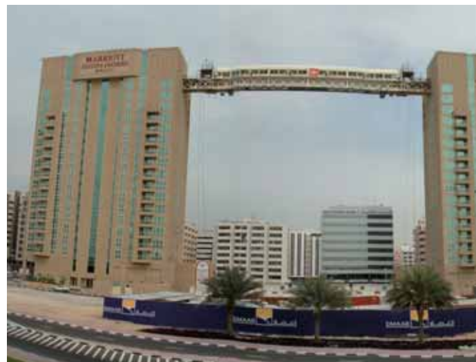
Marriott Apartments, world record sky bridge span, Dubai, UAE Lifting the 56m-long centre part of the 280t sky bridge to the 60m-high level of the 19 th floor.
