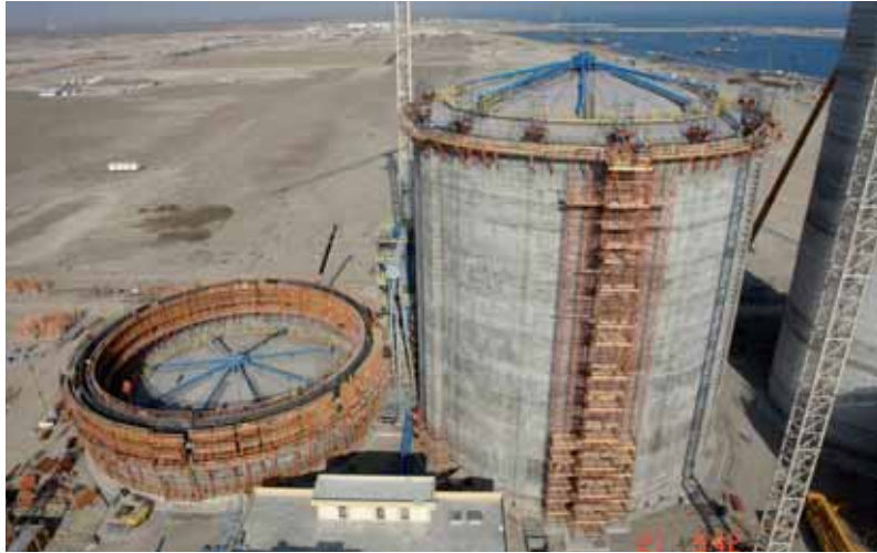
Alumina Silo, Sohar Port, Sultanate of Oman Lifting by 50m of two delicate 250t steel silo roofs.
