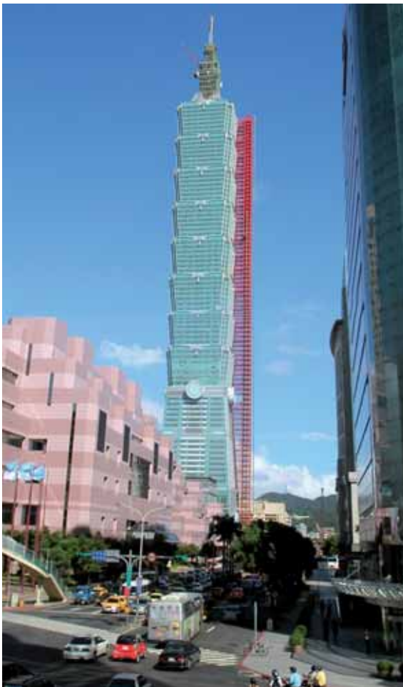
Taipei 101 Building, Taipei, Taiwan Jacking up of the 460t, 60m-long pinnacle from the 60 th floor to top of what was the highest building in the world from 2003 to 2007. Final height: 508m
