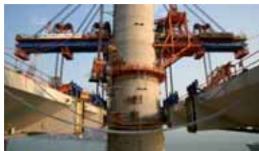
Stonecutters Bridge, Hong Kong Lifting and moving of pier table segments together with simultaneous lifting of a double-deck span at each pylon. Maximum lifted weight: 4,000t, height: 70m.
