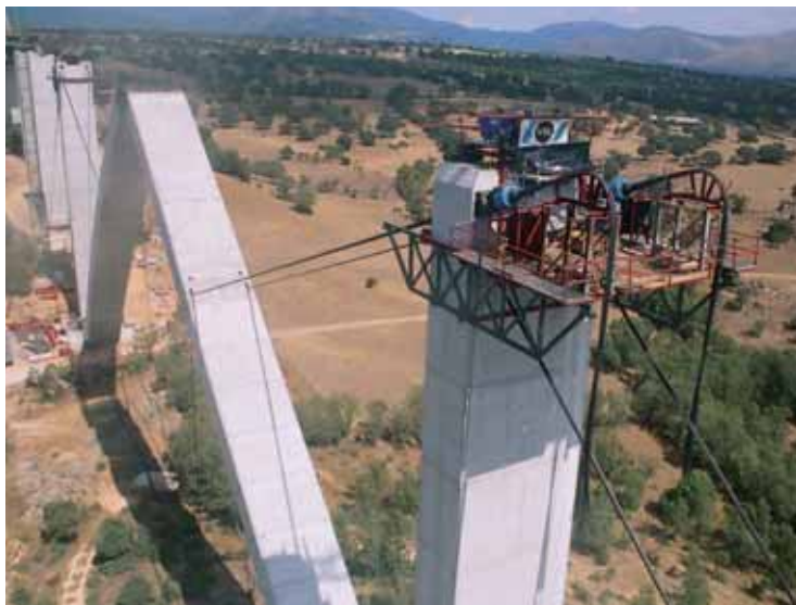
High Speed Railway Miraflores Viaduct, Spain Tilting into final position of 132m support arches. Weight: 1,400t each
