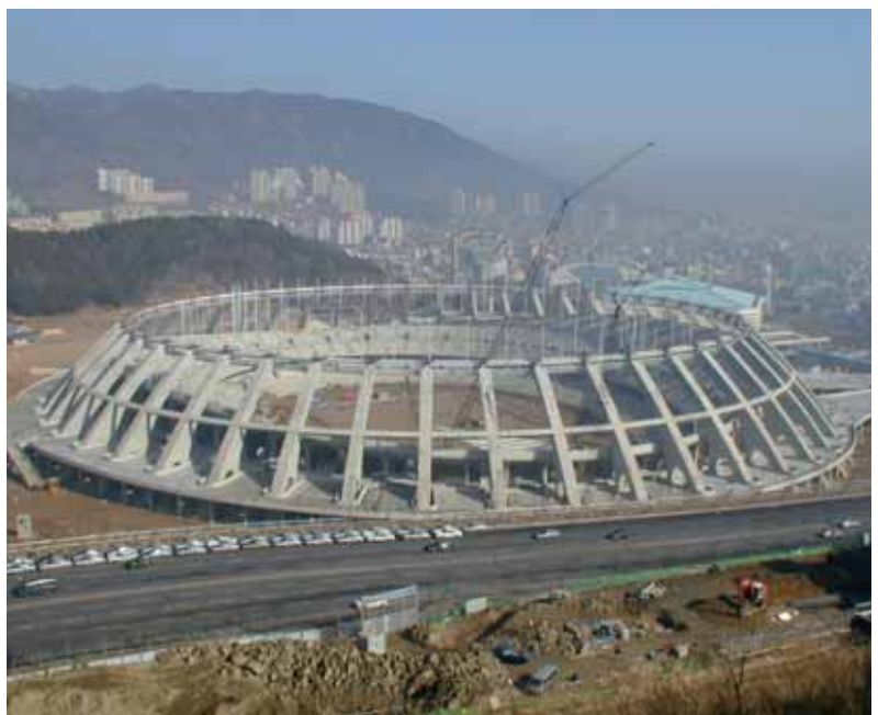
Pusan Dome, South Korea Lifting and tensioning of cable roof with a double tension ring cable and 2 x 48 radial cables. Total installed lifting and pulling capacity: 8,000t
