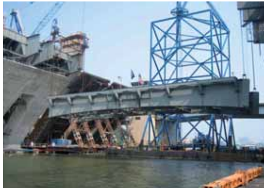
Woodrow Wilson Bridge, crossing the Potomac River at Alexandria, USA Lifting two 500t spans by 40m from a barge. Span dimensions: 47m by 17m each
