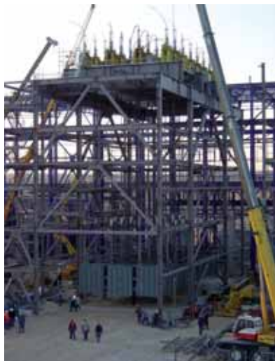
Castelnou CCCP, Spain Lifting of 24 modules for two boiler units. Lifting height: 20m. Weight: 1,800t each
